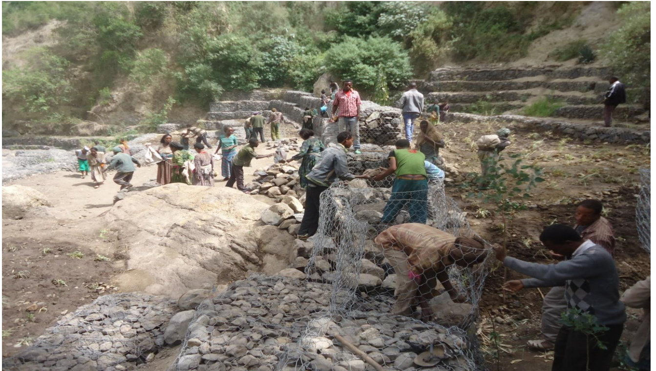
Spring protection, capturing groundwater for use
