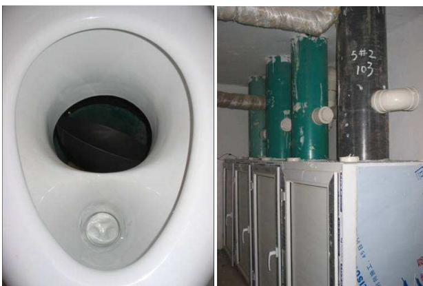
Figure 18. Left : Ceramic urine diverting dry toilet equipped with turning bowl, automatic sawdust supplying device and trap for urine. Right : Downpipes coming from each floor leading into separate bins with housing (Erdos Eco-Town, Dong Sheng, China, photos: W. Berger, 2009)
