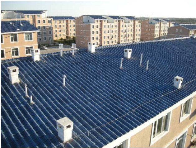
Figure 16. Part view of the multi-story houses in Dong Sheng, showing vent pipes on the roof from the ventilation system (photo : W. Berger, 2009).
