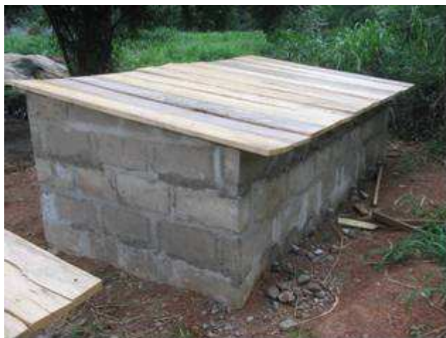
Figure 2. Brick chamber for faeces composting equipped with vent pipes on the back side and sheltered (photo: W. Berger, 2009 at German Research project at Valley View University, Ghana)
