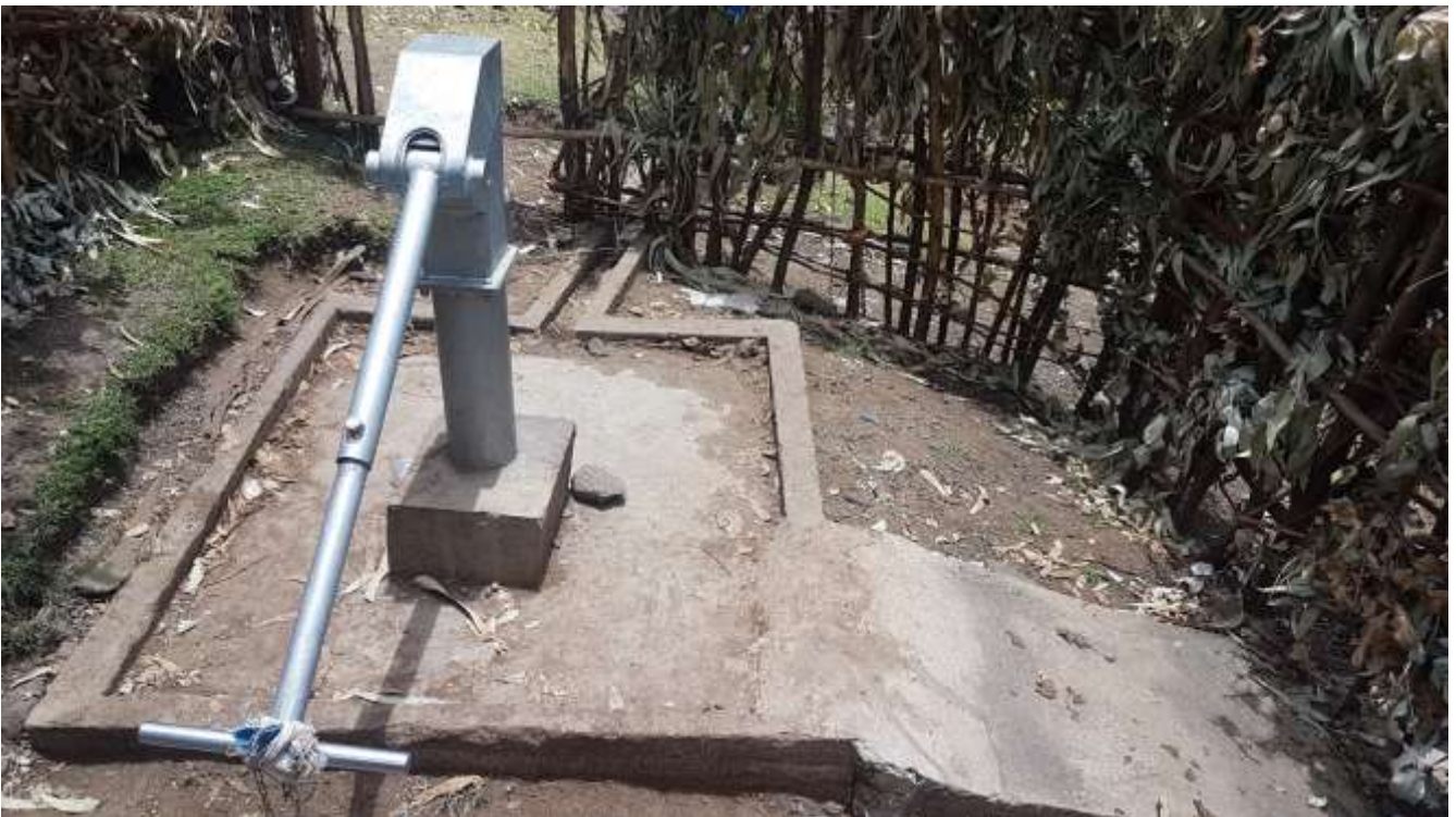
Inaccessible shallow well constructed in 2011 EFY and visited in Ofla woreda
