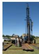
Boreholes equipped with hand pumps or submersible pumps with small distribution network
