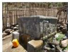
Spring protections with collection chamber and small gravity distribution network with cattle troughs and shower houses
