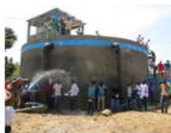
Large multi-village piped systems with motorized pumping, collection chamber and gravity distribution network with cattle troughs and shower houses
