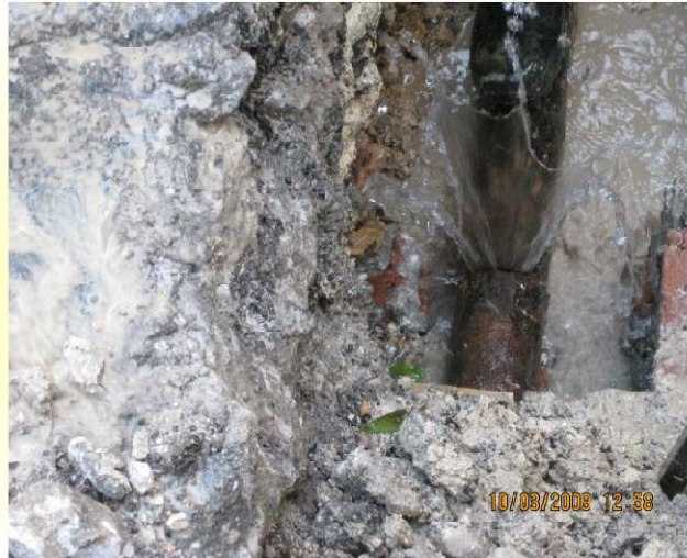
Figure 9: Corrosive attacks of pipes
