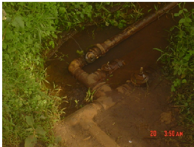
Figure 2: Typical visible leaks from a valve (Durame Picture by MCE)
