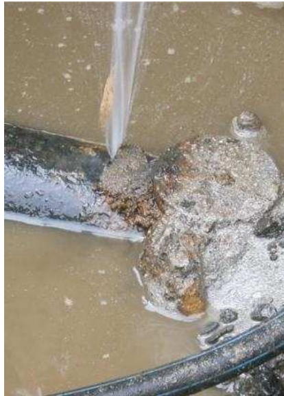
Figure 12: Leakage from an Old Pipe Burst
