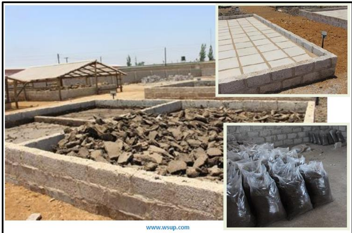
Figure 16: Decentralised pit latrine sludge treatment and commercial sales in Lusaka, Zambia
